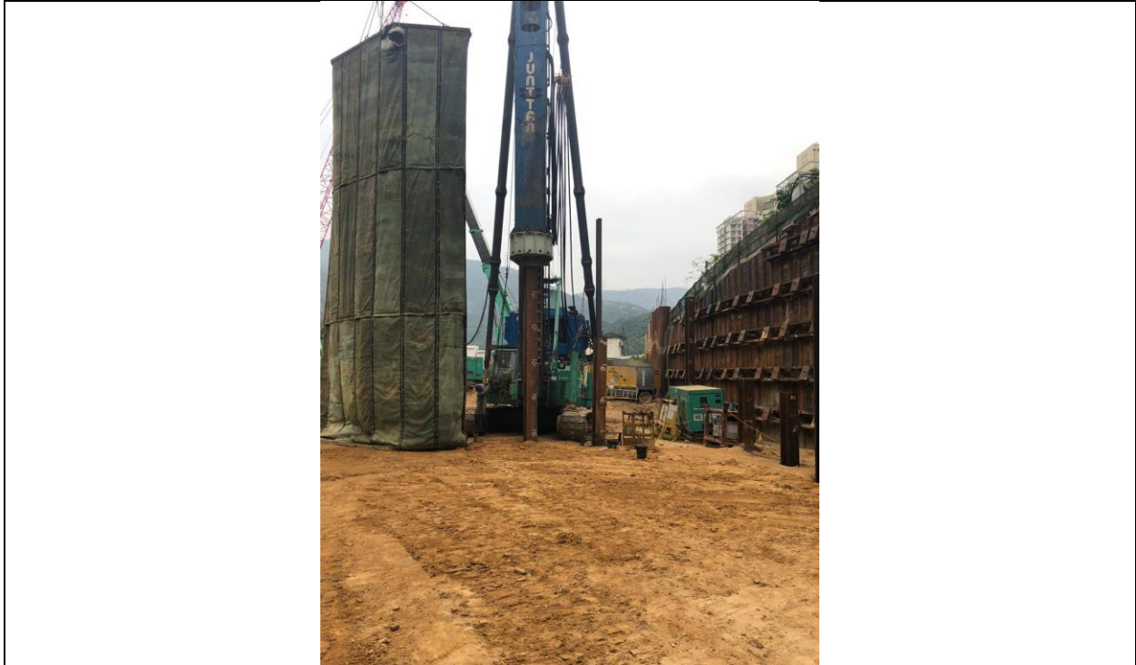
Hoisting of noise barrier during piling 打樁過程中隔音屏障的吊裝 打桩过程中隔音屏障的吊裝
