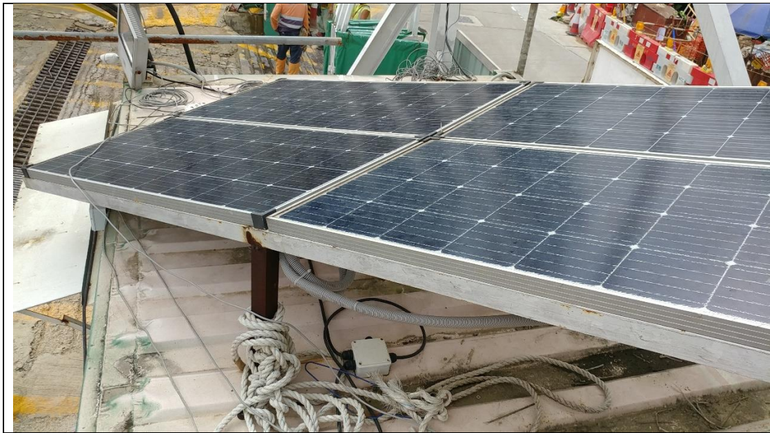
Using solar panel to provide energy for security room.
